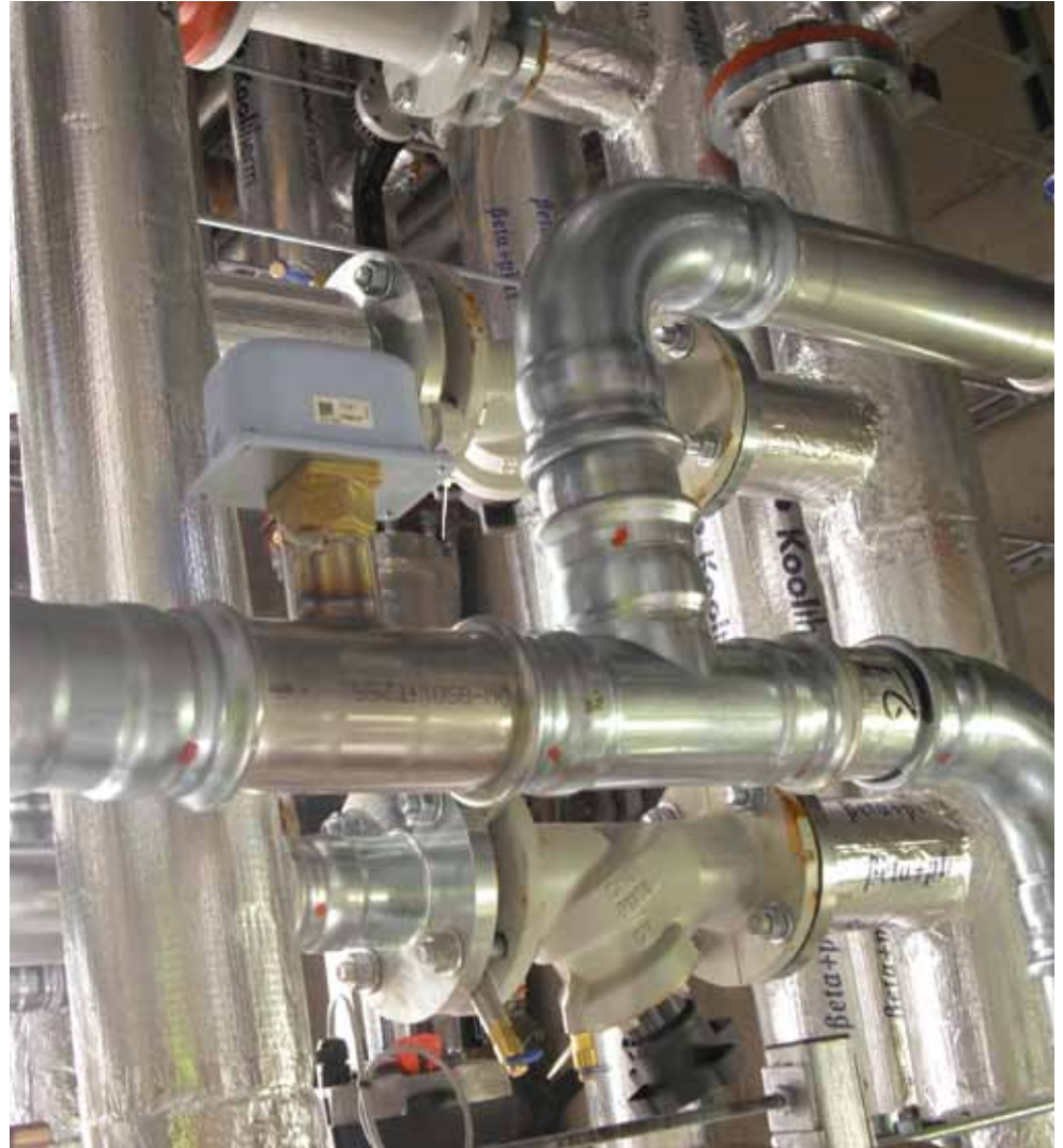
↑ Geberit Mapress Carbon Steel is among a whole host of Geberit products installed in the Hepworth Gallery.
