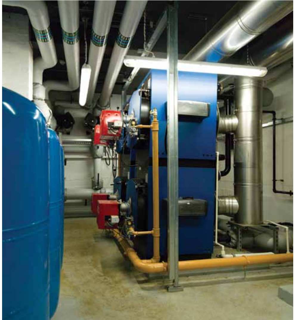
↑ Forest School boiler room, including Two Hamworthy Ansty dual module boilers with Riello burners, rated at 249kW each.
